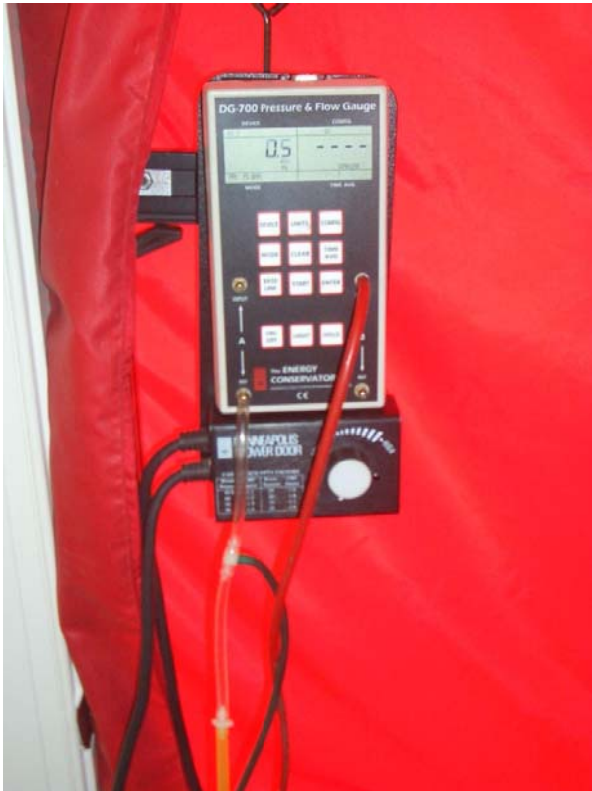
Figure 3 Monometer set up for unit 1204
